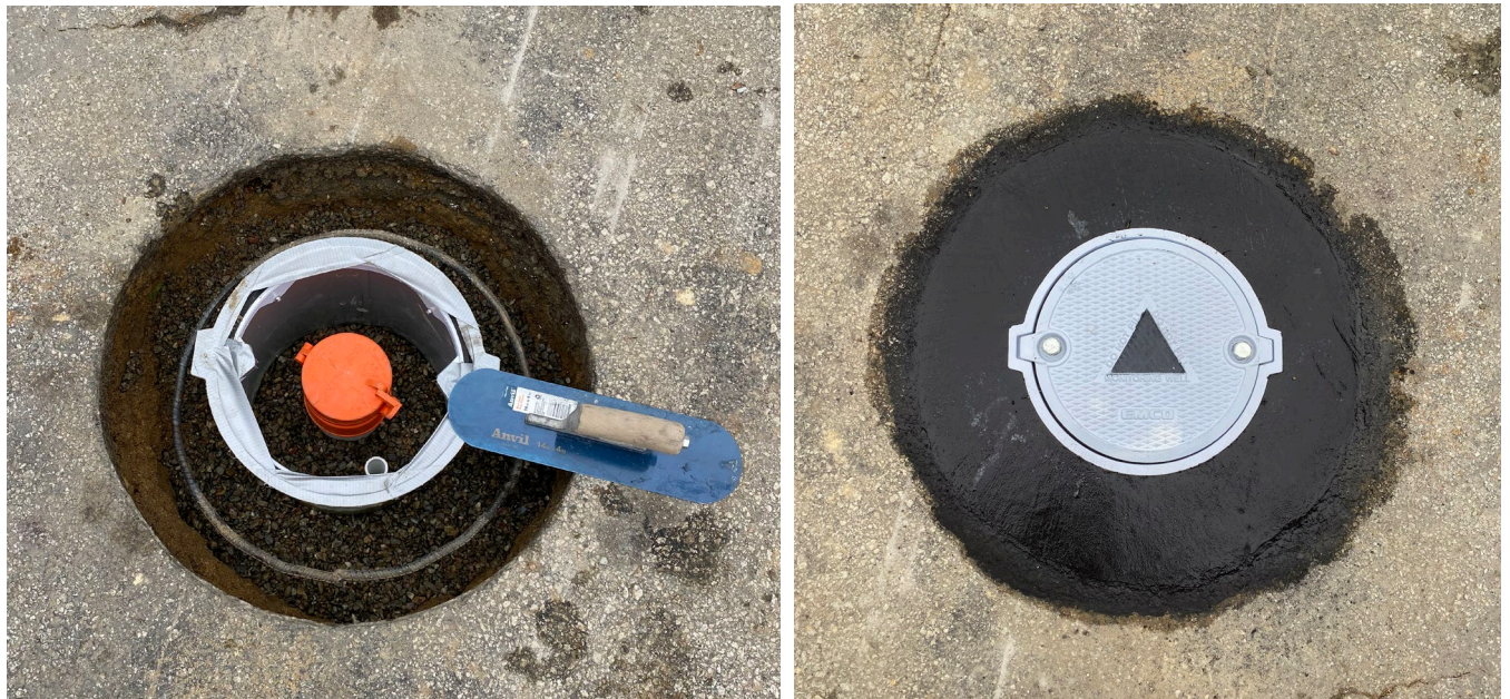
Figure 10. Example Well Vault Installation at SGMWA-5 Bahr Drive
