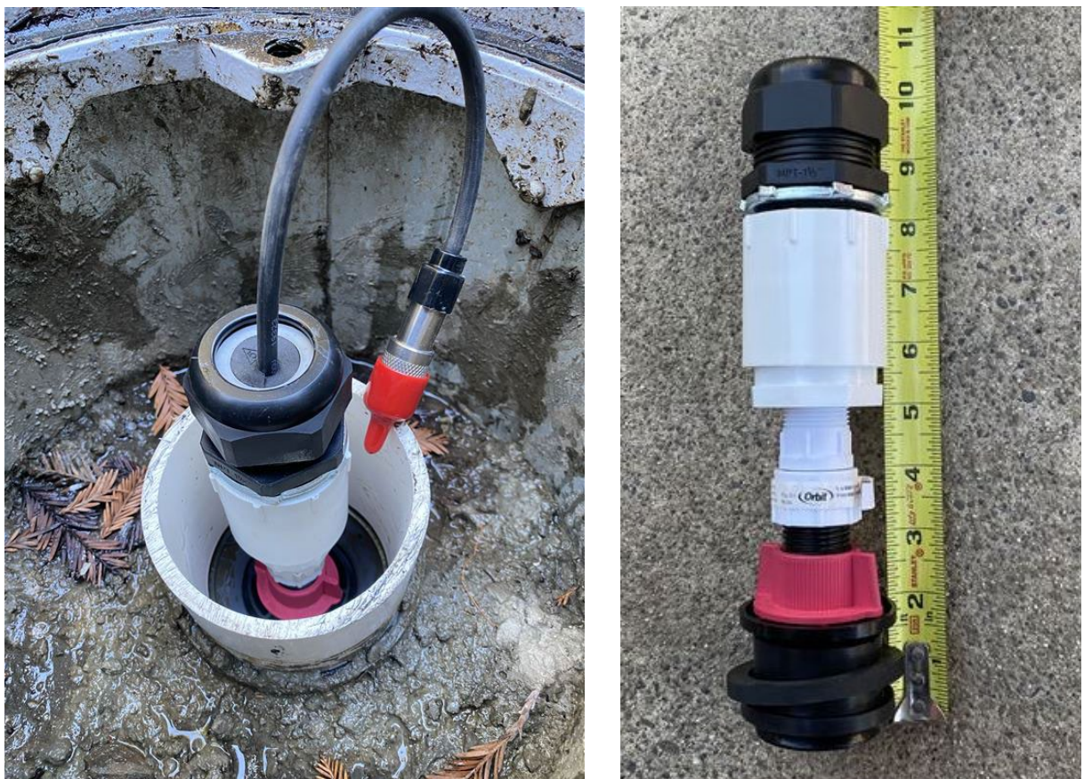
Figure 14. Transducer Equipping and Artesian Wellhead at SMGWA-7 Love Creek
